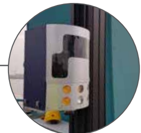
A pair of facing BoxCatcher cameras is mounted onto vertical guide rails, attached to the STS portal legs
